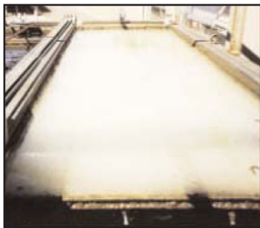
The Clari-DAF System Creates a milky solution of hundreds of millions of microbubbles 20 to 100 microns in size that rapidly float suspended particles to the surface for removal
